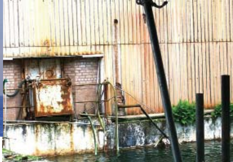
Rust, corrosion, and weeds growing in cracks in the concrete walls of nuclear waste storage ponds at Sellafield.
