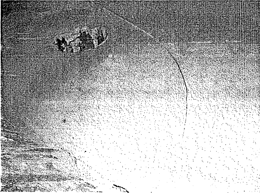
Bay 19 floor separation left side
