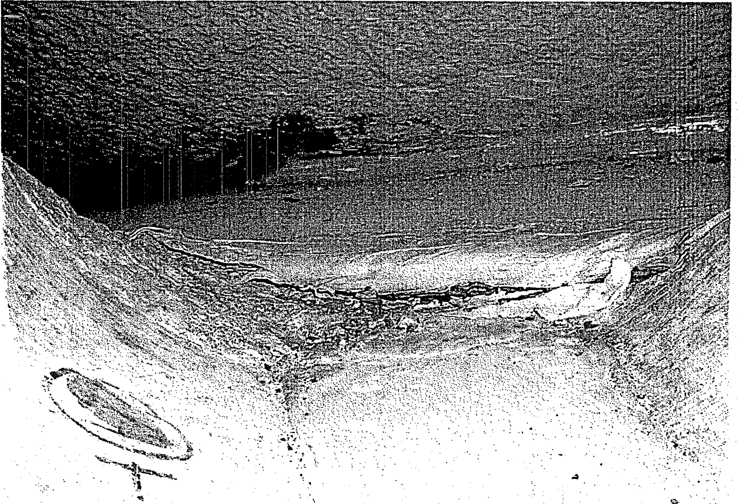
Caulking build-up at manway entrance.
